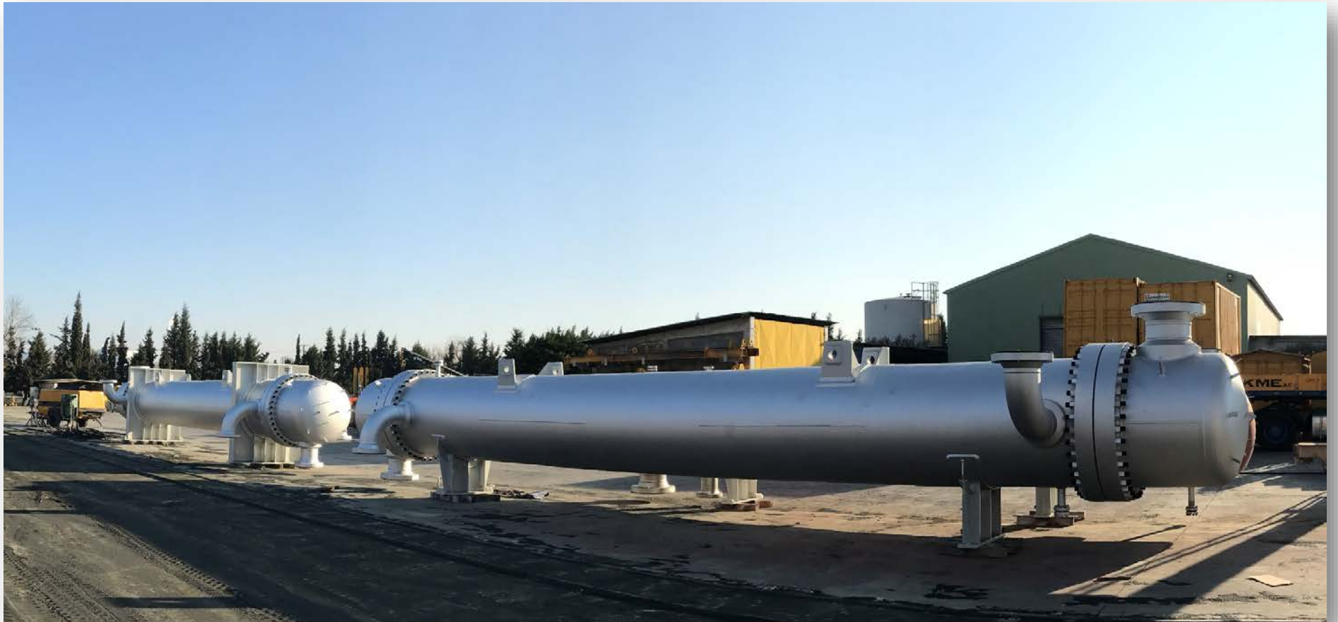
010-E-311 1/2 Gas-Gas Exchanger (1st & 2nd Shell)
