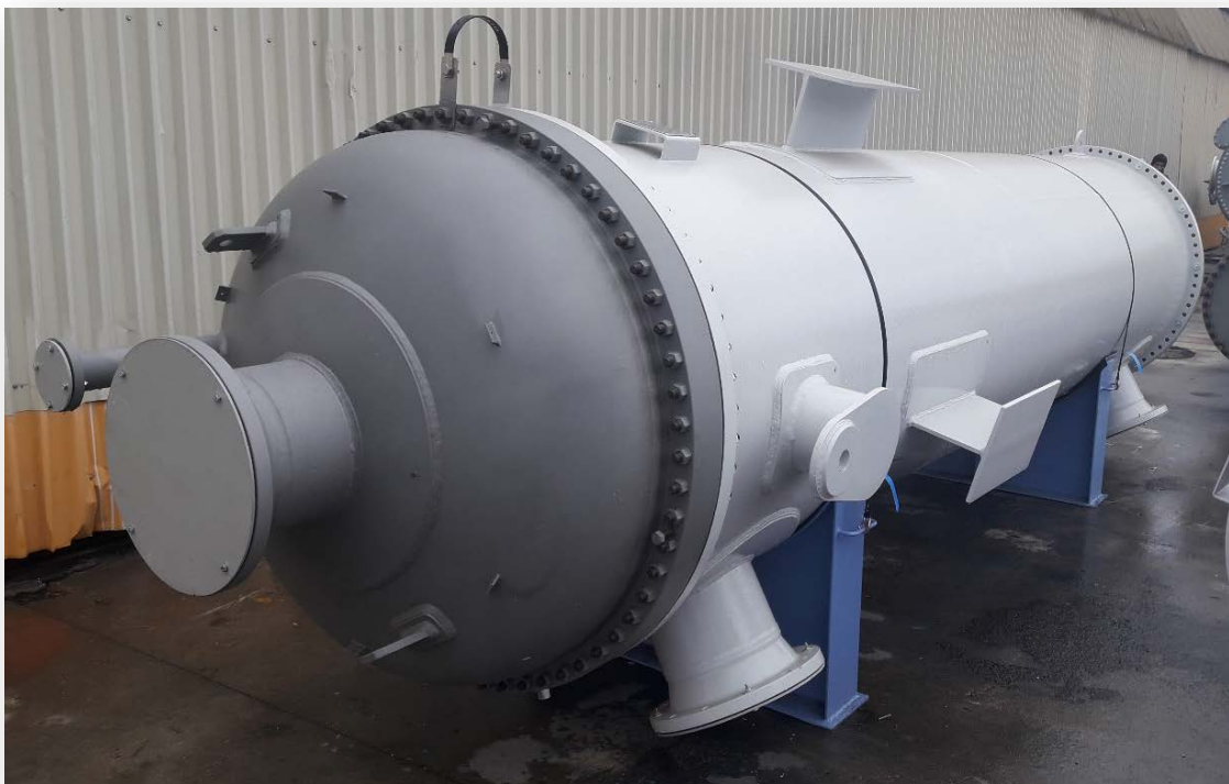
E-3005 Intermediate Treatment Scrubber Condenser
